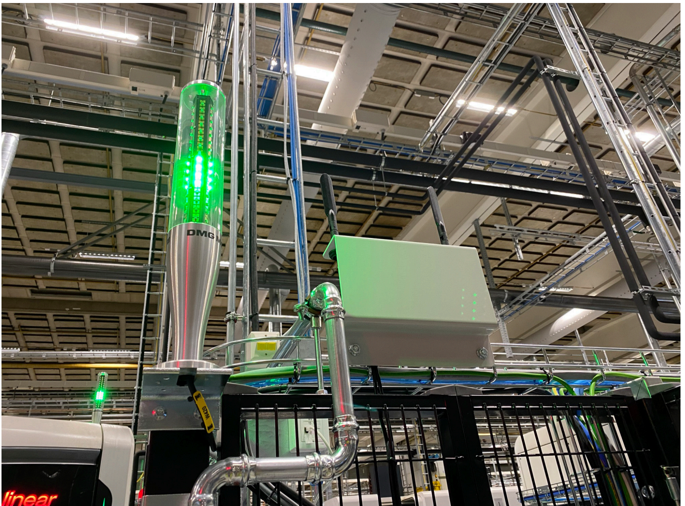
The Anybus Wireless access points, with Mesh capabilities, provide excellent network coverage and seamless roaming throughout the production area.
